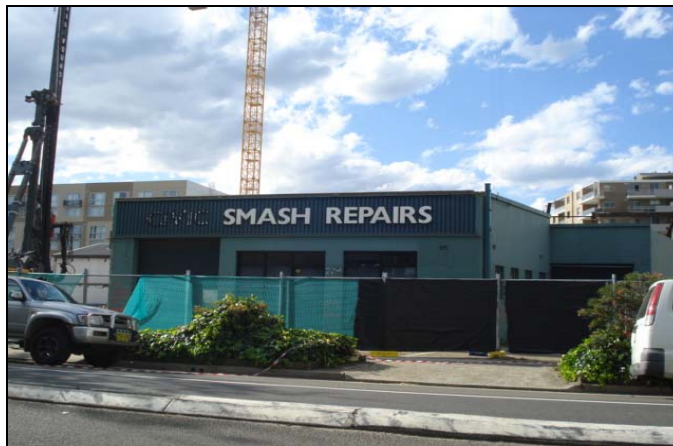
Subject site as viewed from Coward Street. Note: Buildings have been demolished.
